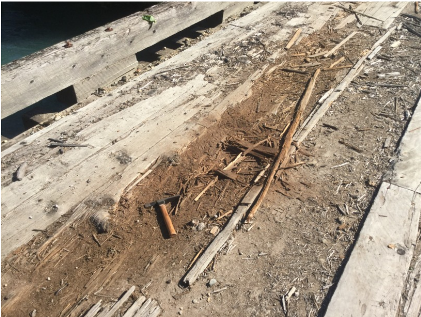
Rotten Running Strip
