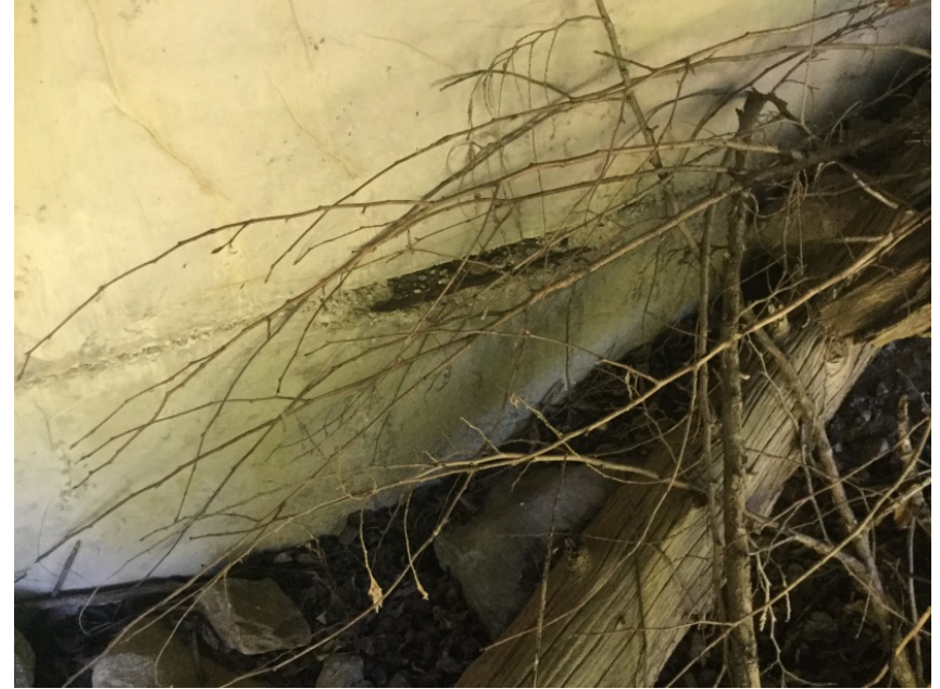
Spall with Exposed Rebar Right Abutment
